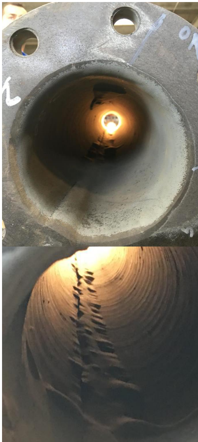
Figure 1.3 Non-performing Bubbles arising between Body and Lining of the Abu Qir Fertilizer Plant
