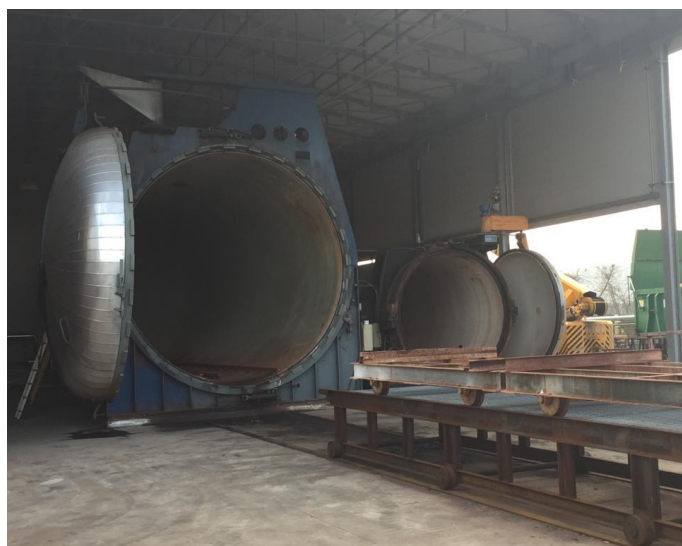
Figure 1.7 Rubber is finally fixed through the Vulcanization method
