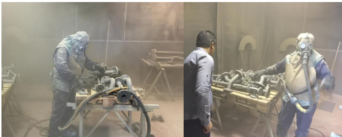
Figure 1.5 Damaged Pipes are cleaned and restored through Heating, Air Flushing and Sandblasting processes
